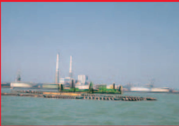
... and delivers it through a floating pipeline to gravel spraying pontoon BAYARD II
