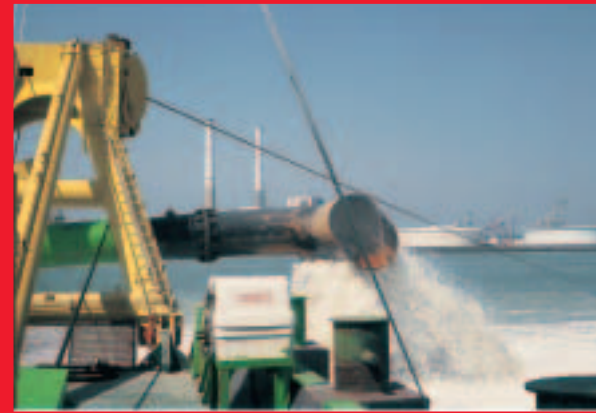
The spray pipe is lowered under water only when gravel production starts
