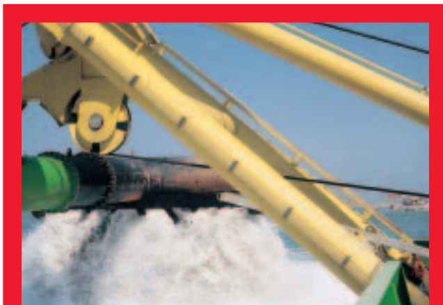
The gantry, delivered by IHC E&R, keeping the spray pipe at 6.30m aside the BAYARD II
